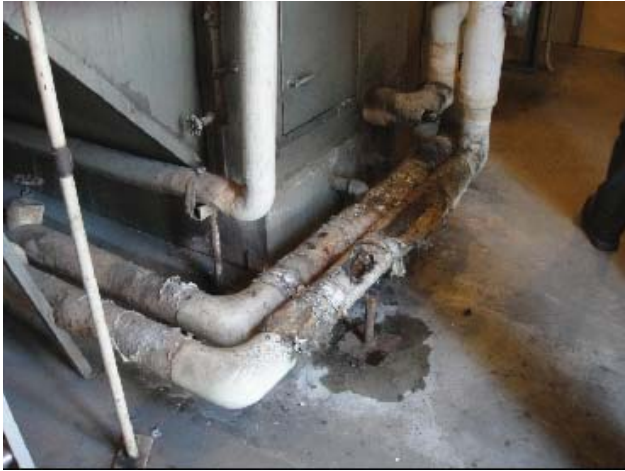
Figure 13: Rusty Piping and Deteriorated insulation
