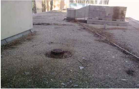
Figure 22 - Corroded Storm Drains on the Roof
