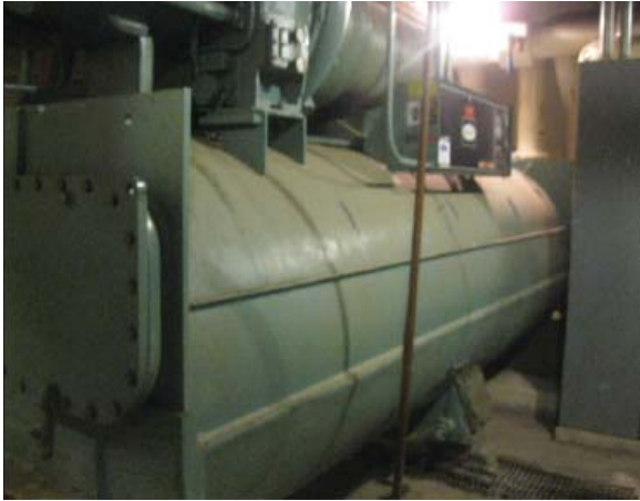
Figure 6: 300 Ton Centrifugal Chillers
