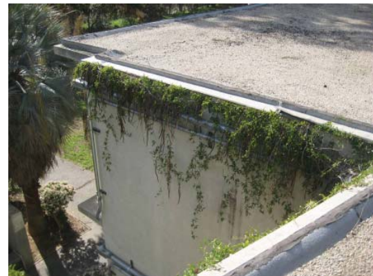
Photo 18 Vegetation growing in the gutter at the perimeter of Building B.
