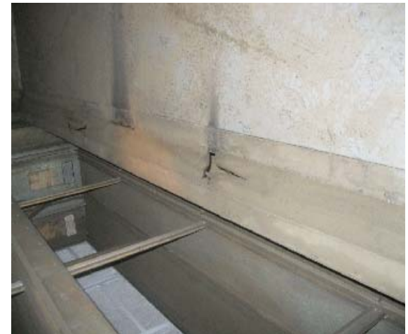
Figure 8: Flexible Connection Broken on Most AHUs
