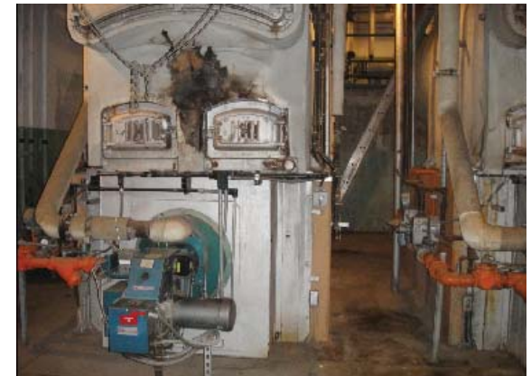
Figure 2: 13,650 MBH Steam Boilers in the Basement
