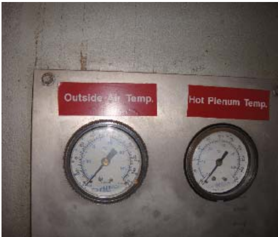
Figure 10: Nonworking Instrument on Control System
