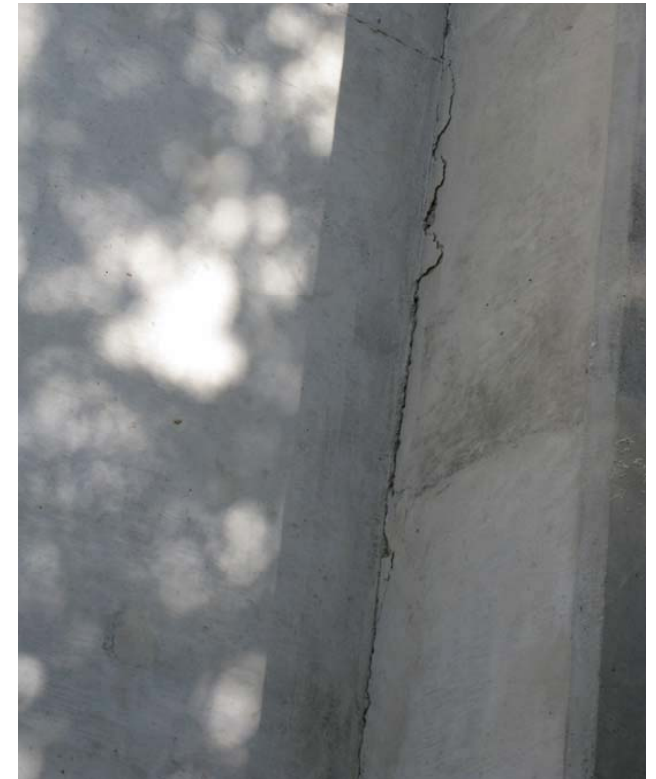
Figure 4: Closeup of Crack in Wing D West at Gridlines K-1
