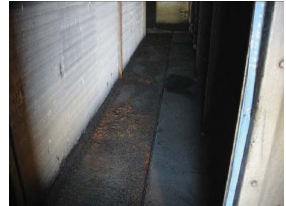
Figure 7: Rusty Baseplate Found on Most AHUs
