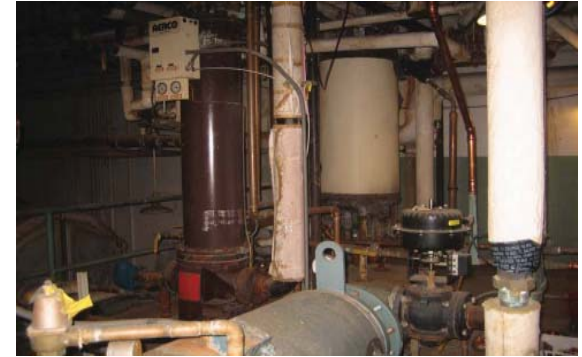
Figure 23 - Existing Domestic Hot Water Heat Exchangers
