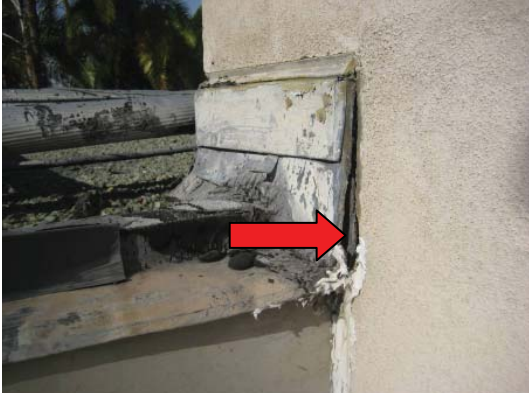
Photo 14 Flashing at the transition between an upper roof and lower roof. Note the opening between the flashing at the wall (arrow).
