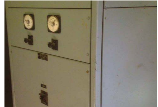
Figure 16 - Main Switchboard for the 300 KVA, 208/120 V Unit Substation Serving the General Power and /Lighting of Building C
