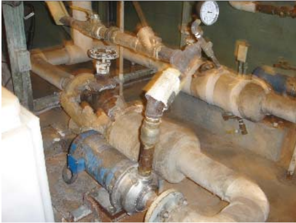
Figure 3: Pumps of Steam Heating System in the Basement
