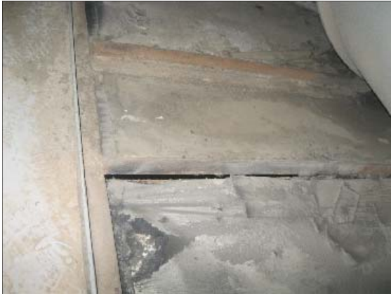
Figure 9: Crack on Baseplate of AHU (Building A West Wing)
