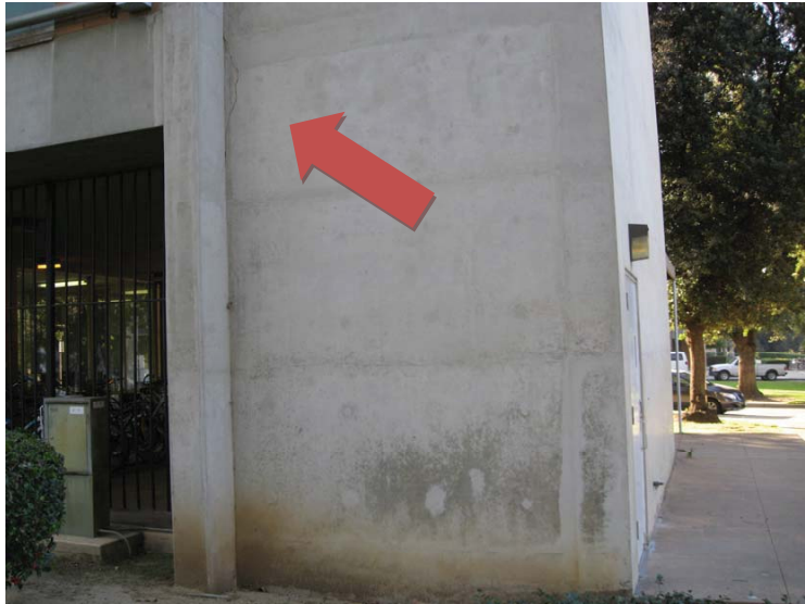
Figure 1: Crack in Wing B West at Gridlines A-1
