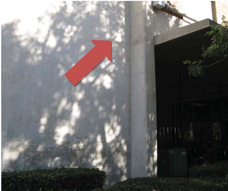
Figure 3: Closeup of Crack in Wing D West at Gridlines K-1
