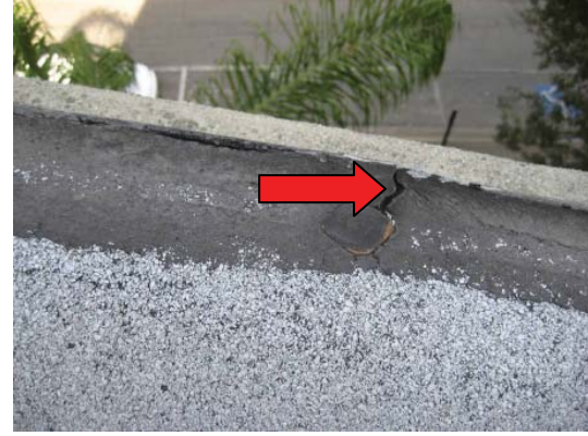
Photo 16 Thin layer of roofing membrane over fasteners (arrow) at the perimeter of the roofing. Note that the membrane is cracked adjacent to the fastener and that the fastener is corroded
