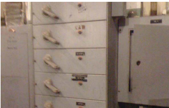
Figure 20 - Typical Motor Control Center, Operational but Beyond Its Service Life
