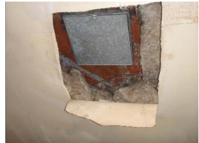
Figure 12: Rusty Duct, Broken Insulation and No Label to Fire Damper
