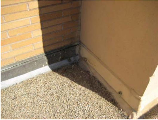
Photo 13 Reglet-set counterflashing (brick side) and surfaced-mounted counterflashing (plaster side) at the perimeter of the roofing membrane.
