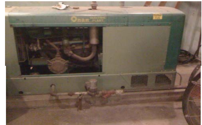
Figure 17 - 25 KW, 120/208 V Natural Gas Fueled Emergency Generator
