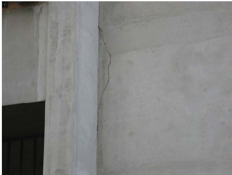
Figure 2: Closeup of Crack in Wing B West at Gridlines A-1
