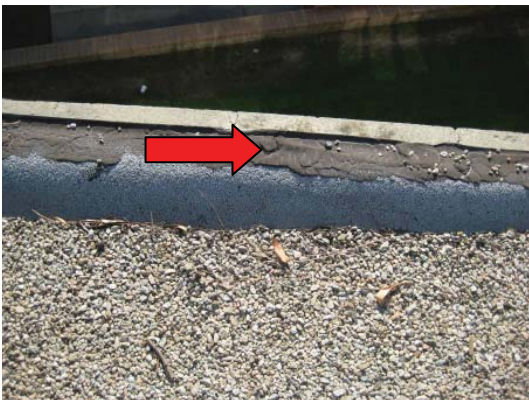
Photo 15 Thin layer of roofing membrane over fasteners (arrow) at the perimeter of the roofing.
