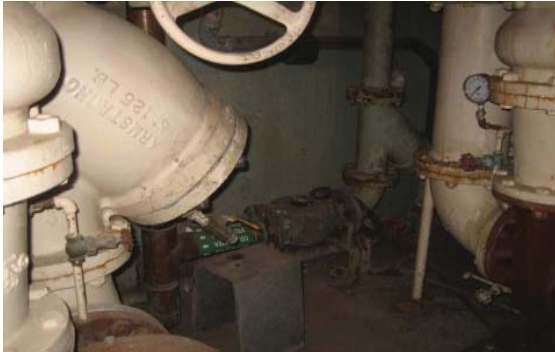
Figure 24: The Incoming Main and Meter in Need of Replacement
