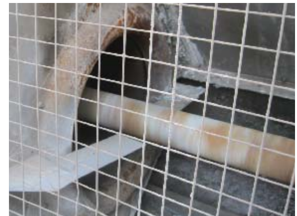
Figure 5: Cooling Tower in Rusty Condition
