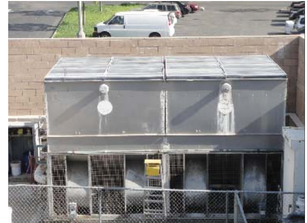
Figure 4: Cooling Tower in the Courtyard of Loading Dock
