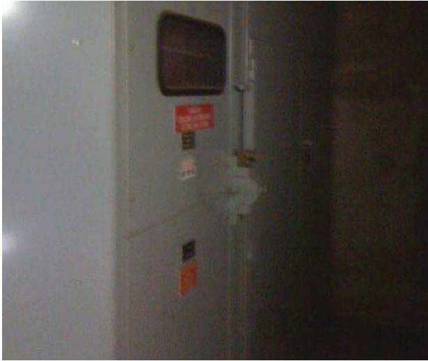
Figure 15 - The 750 KVA, 480 V Unit Substation Serving the Chillers, Boilers, and Pumps
