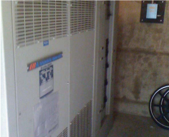
Figure 18 - Typical Building 300 KVA, 208/120 V Unit Substation
