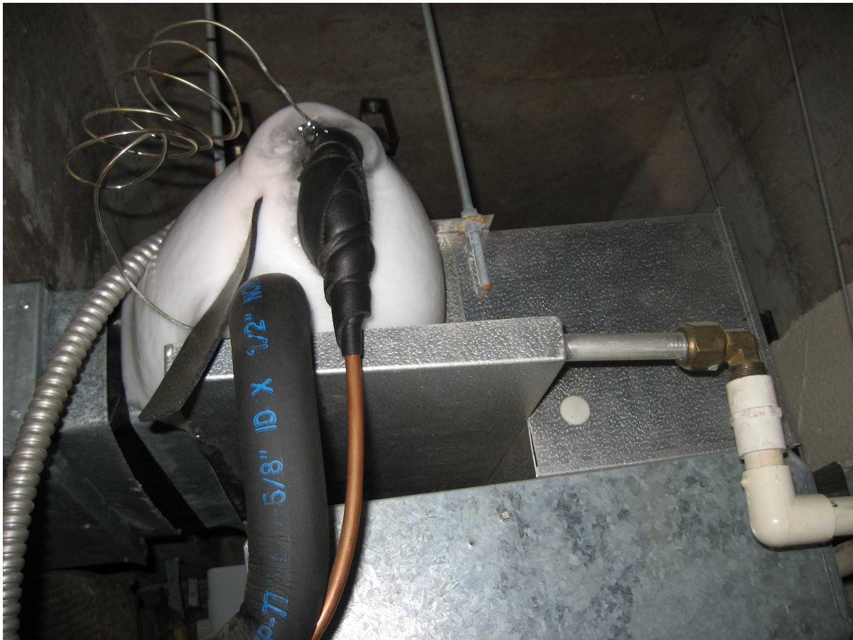
Figure 3-9: Ice block at Fan Coil Unit FCU-1 in Room 2690
