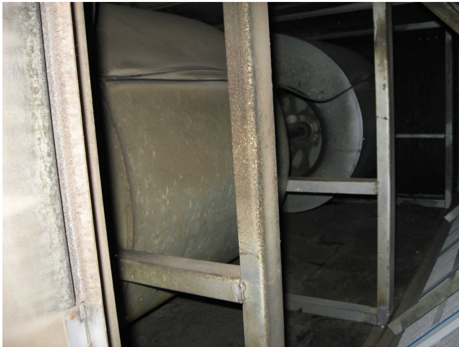
Figure 3-1: Existing Supply Fans in AH-2
