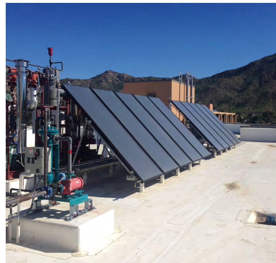
Existing solar thermal PV installation at Glen Mor
