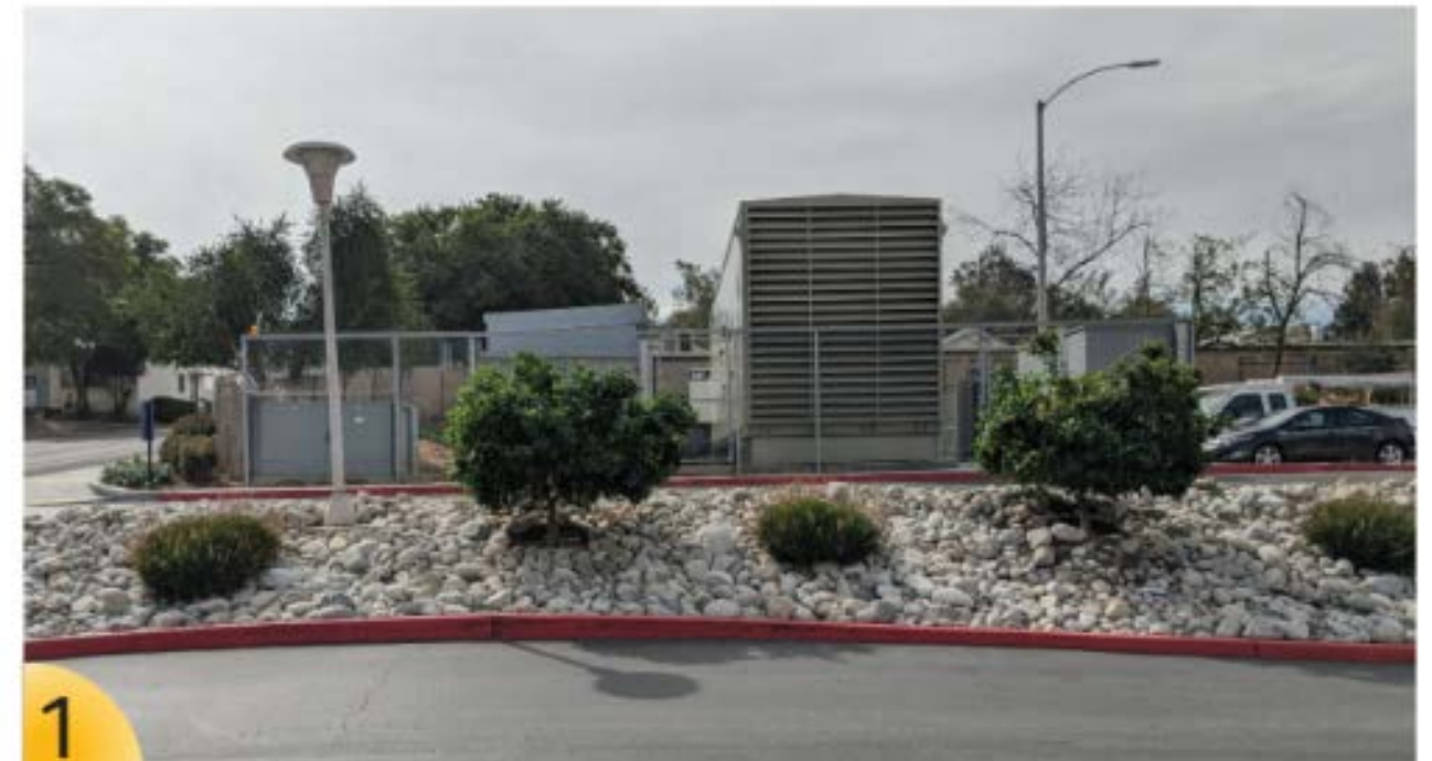
ELECTRICAL EQUIPMENT TO BE REPURPOSED AND RELOCATED ON SITE
