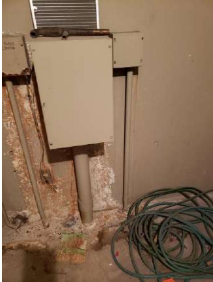
View of Gray Metal Pipe
