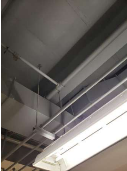
View of Dark Gray Metal Pipe
