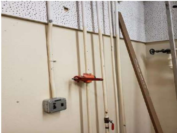
View of Off White Metal Pipe
