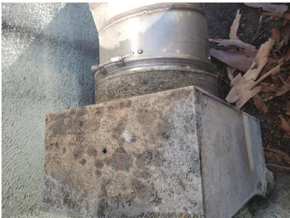
View of Gray Transite HVAC Inlet Box
