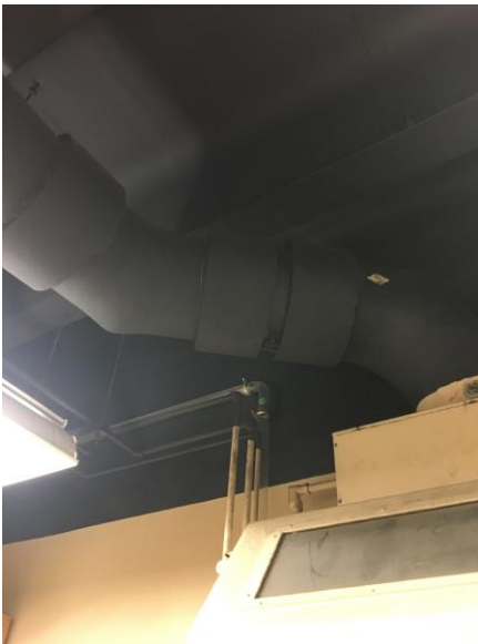
View of 24" Transite Fume Exhaust Pipe
