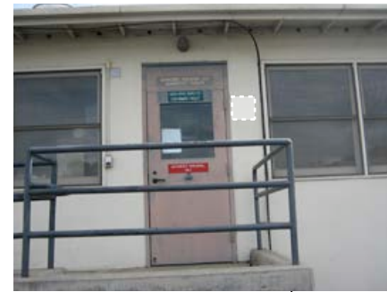
Replace with W52 Wall Mounted Bldg ID
