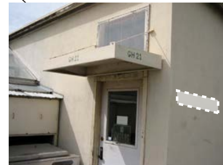
Replace with W52 Wall Mounted Bldg ID
