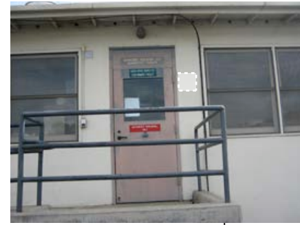
Replace with W52 Wall Mounted Bldg ID
