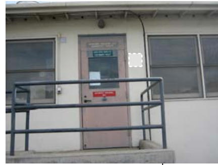
Replace with W52 Wall Mounted Bldg ID
