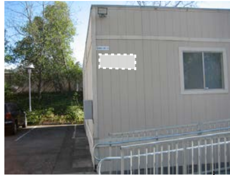
Replace with W52 Wall Mounted Bldg ID
