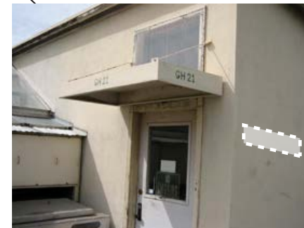
Replace with W52 Wall Mounted Bldg ID
