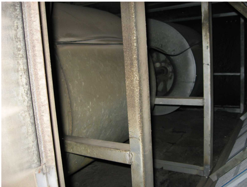
Figure 3-1: Existing Supply Fans in AH-2
